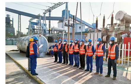
▲ 为110kV变电站提供检修服务 Provide the overhauling service for 110kV power substation
